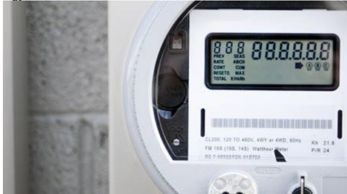
Fig 8: AMI is the calculation of energy cost and the real-time notification of inhabitants [31].
